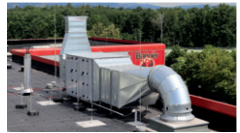
Fig. 12 Dry filter plant
